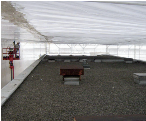
Installation of an internal lining for a decommissioning operation – STED Grenoble – February 2010
