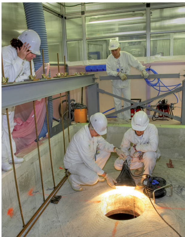
Cleaning out a tank in the vitrification shop of Marcoule – August 2007
