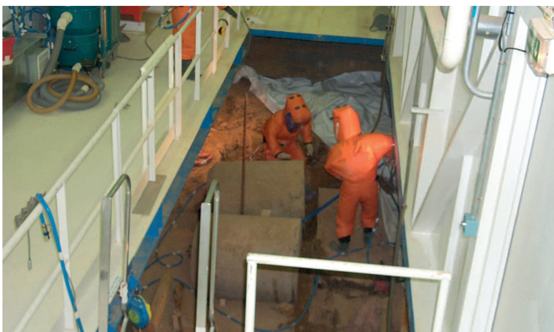
Operators working on the recovery of waste from the trenches of BNI 56 in Cadarache (Bouches-du-Rhône département)
