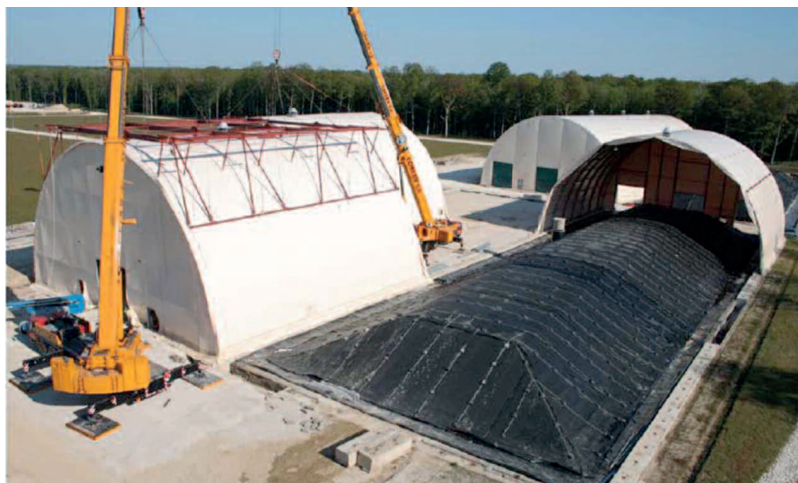
Operations to close cells and move the mobile roof on the Morvilliers site (Aube département)
