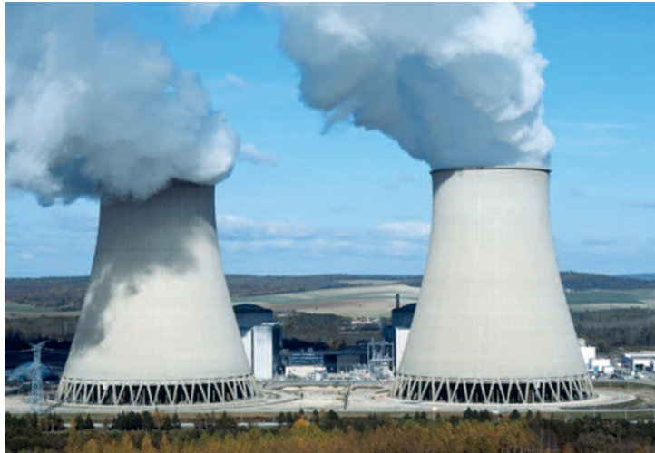
Cooling towers of the Nogent-sur-Seine nuclear power plant: the aerosols are liable to contain legionella
