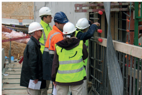
ASN inspectors carrying out an inspection on the MAGENTA facility construction site
