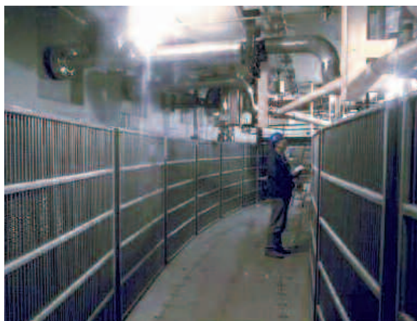
Recirculation sump filter
