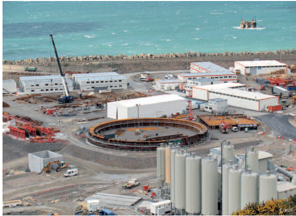
EPR construction site in Flamanville (Manche département) – March 2008: in-situ assembly of the reactor containment internal metal liner
