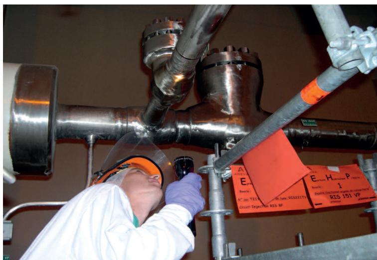
Piping check by an ASN inspector during the primary system hydrotest (Cattenom in the Moselle département ) – June 2008
