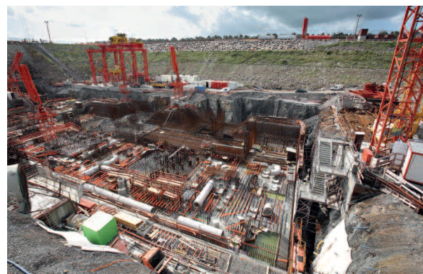
EPR construction site in Flamanville (Manche département) – September 2008: construction of the pumping station
