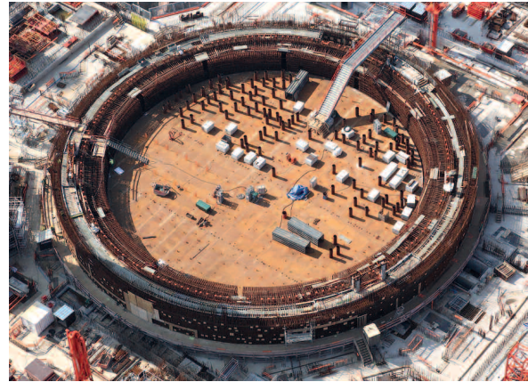
EPR construction site in Flamanville (Manche département) – September 2008: construction of the reactor building with its internal metal liner
