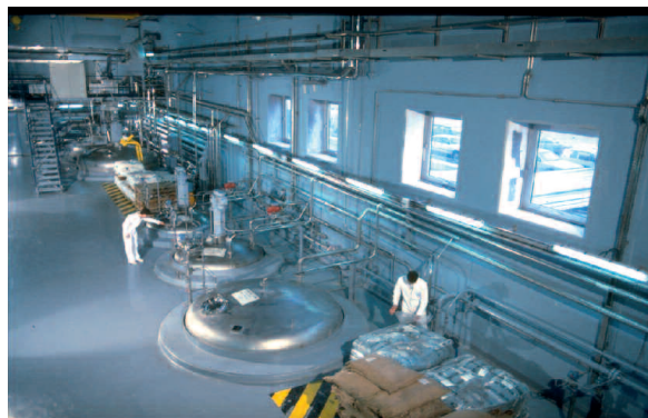
Reagents hall in the STE3 effluents treatment station – AREVA NC at La Hague (Manche département) – 2006
