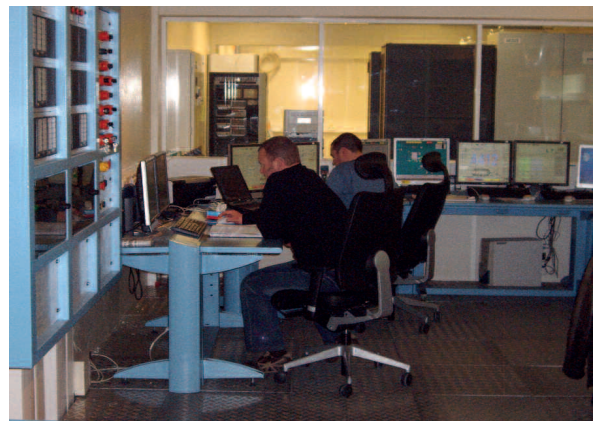
Conversion control room after modification – November 2008
