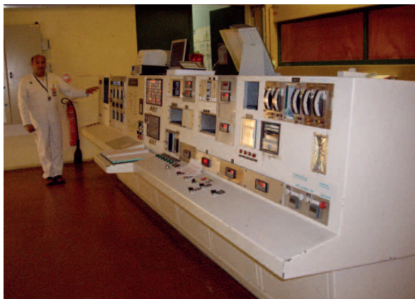
Conversion control room before modification – August 2007
