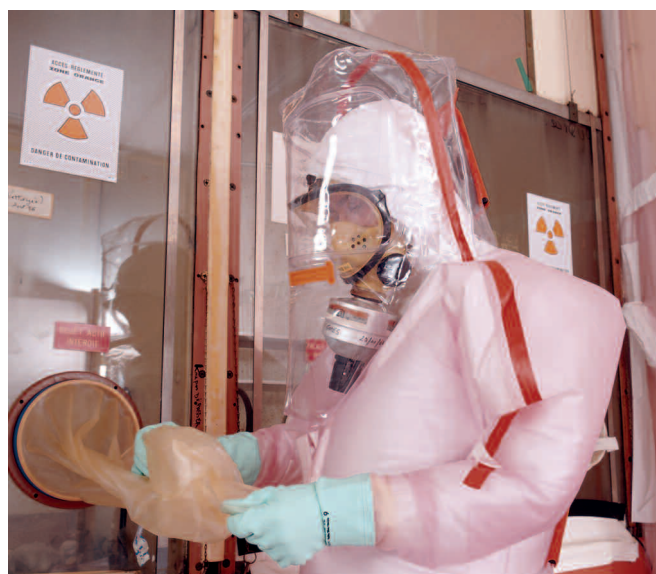
Decontamination of the plutonium chemistry laboratory in Fontenay-aux-Roses (Hauts-de-Seine département ) by an operator in a ventilated vinyl suit with respiratory protection
