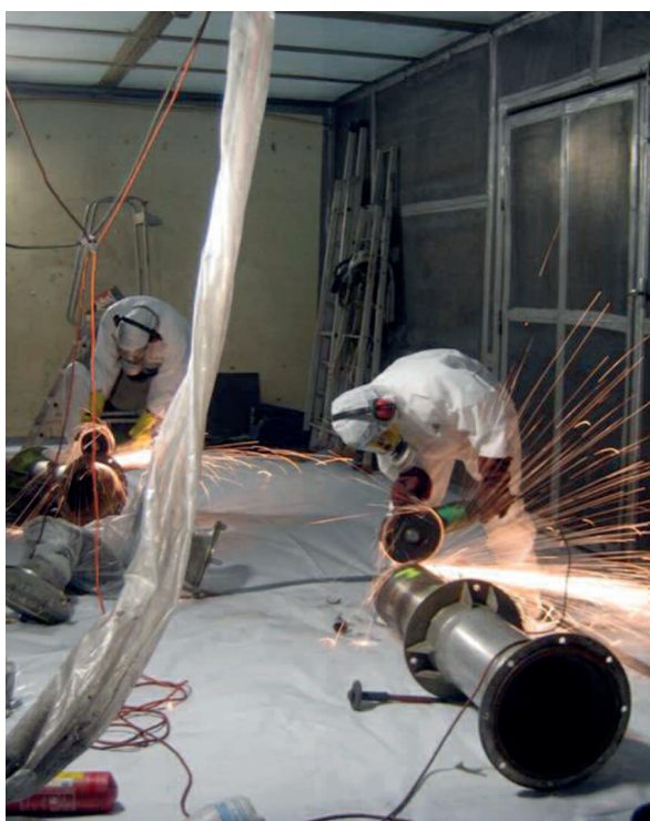
Operators carrying out cutting operations during decommissioning of the ATUE in Cadarache (Bouches-du-Rhône département)
