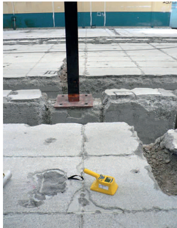
Nuclear installation at La Hague (Manche département) on which complete clean-out operations have been performed
