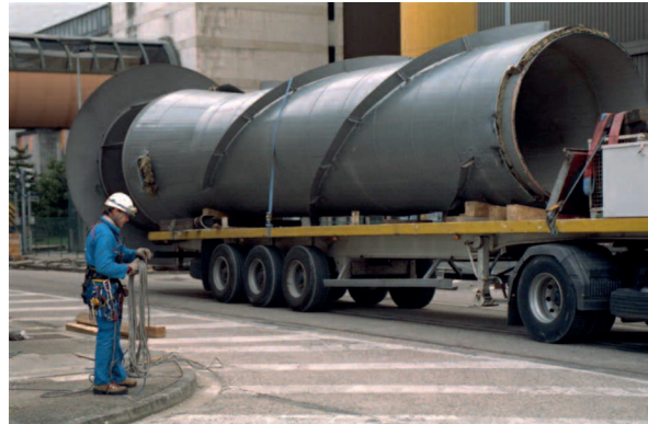
A stack section being placed on a semi-trailer during decommissioning of the SUPERPHÉNIX reactor (Isère département)
