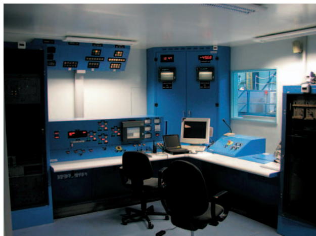
Minerve reactor control room
