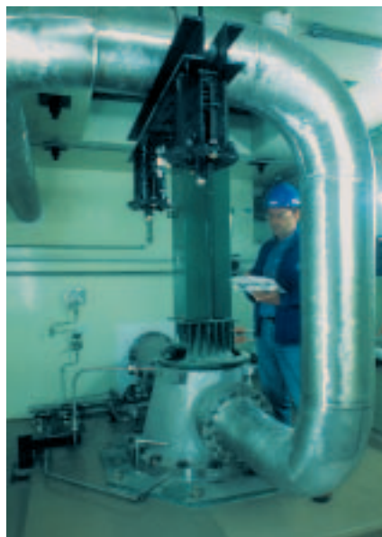
RIS safety injection pump
