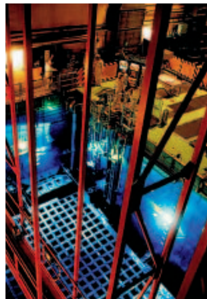
Spend fuel pool at the Saint-Laurent nuclear power plant
