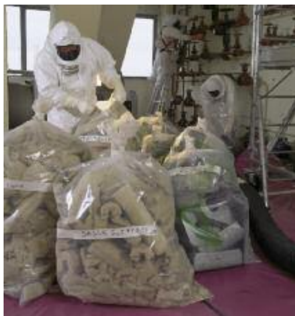
Decommissioning of the Brennilis power plant, shut down since 1985 – removal of pipe lagging in room 605 of the effluent treatment station – January 1998
